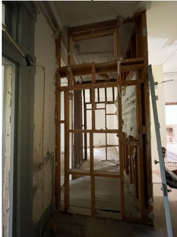
Separating wall between flat and communal area stripped back to the studs
