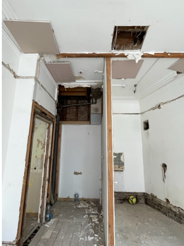
UGF flat to the right stripped with large and plaster construction exposed in areas
