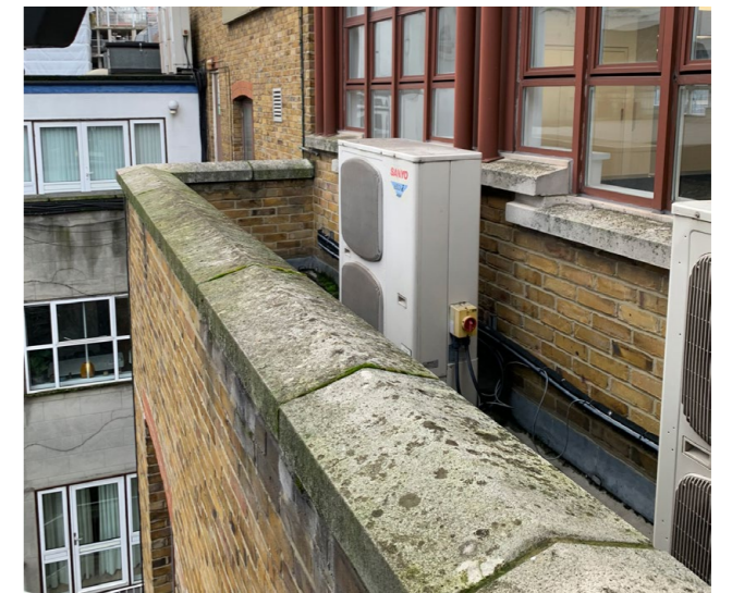
Existing plant arranged across the rear elevation
