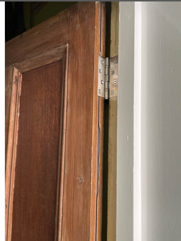
17.17.1 not a notional fire door
