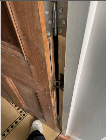
17.17.1 not a notional fire door
