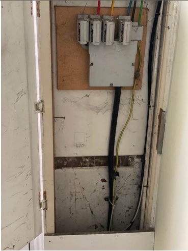
17.20 Ground floor electrical installation
