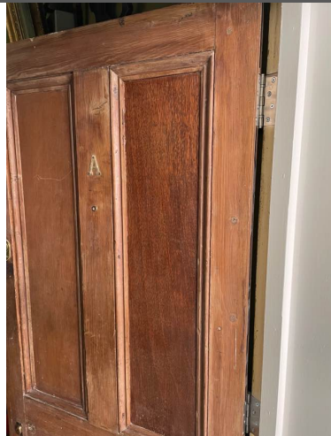
17.17.1 not a notional fire door
