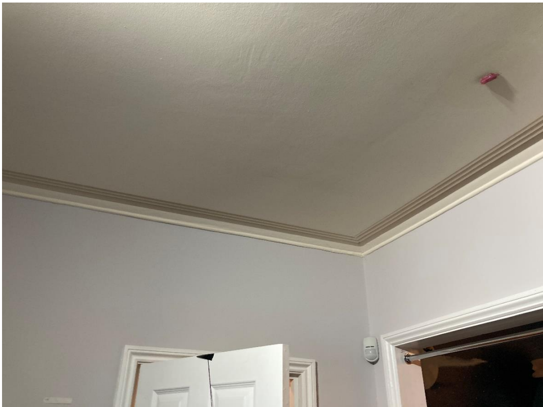
Figure 21: Original Beaded Cornice to Ground Floor Front and Rear Room, with Approved Dry Lining
