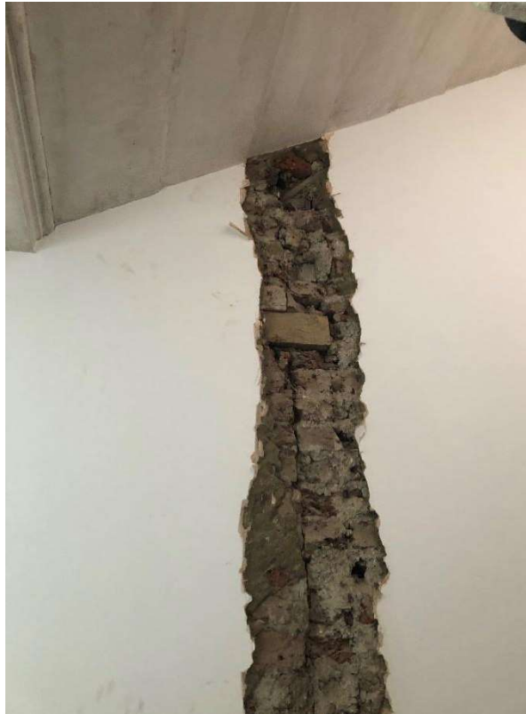
Figure 4 - Opening up has shown a straight crack between two panels of masonry, image 1 of 2
