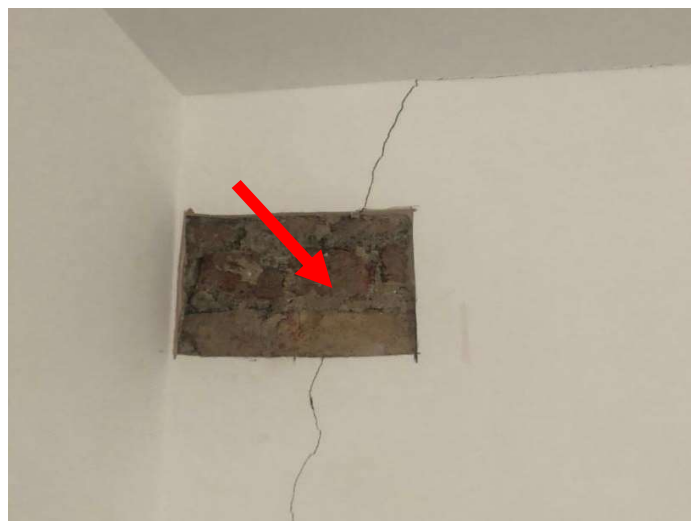
Figure 6 - Removal of the finishes over the crack in the 3 rd floor bedroom wall shows no sign of affecting the masonry structure
