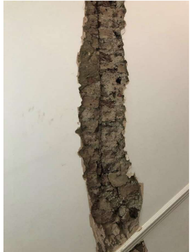
Figure 5 - Opening up has shown a straight crack between two panels of masonry, image 2 of 2
