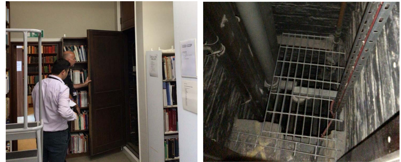
Figure 17 Two pictures showing one of the riser shafts in the Library Reading Room on the third floor.
