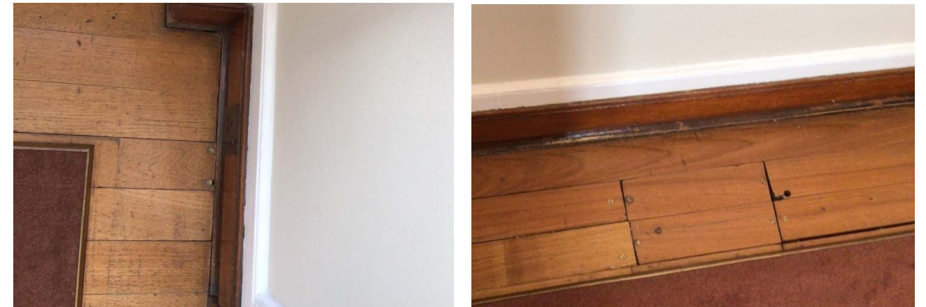
Figure 16 Two pictures showing the teak floors are potentially able to be opened.
