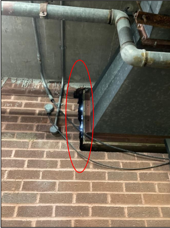
Figure 24 Entry points around metal ducting and louvre doors.
