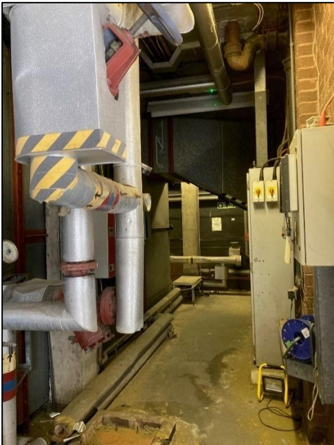
Figure 21 Interior of the boiler room, lit and open
