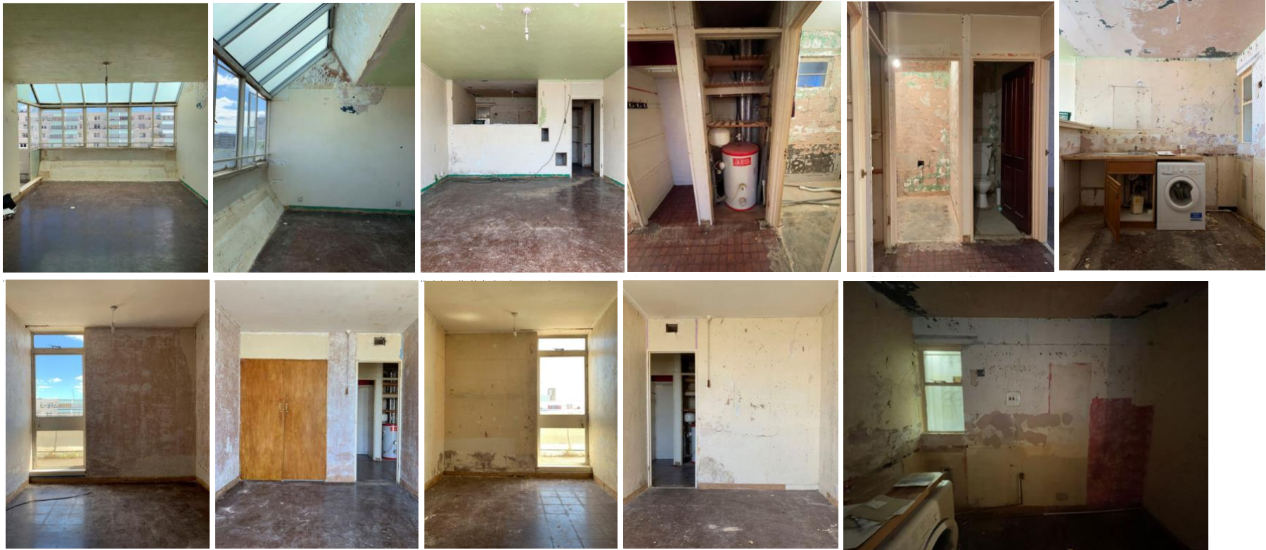
Figure 3: The state of the flat when acquired by the client, prior to asbestos removal.
