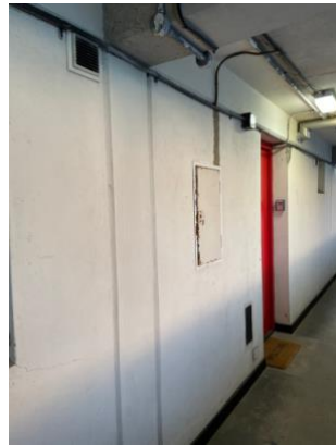
Flat 82 Foundling Court 2 additional grills
