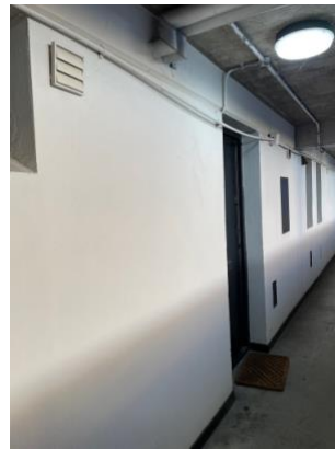
Flat 143 Foundling Court 3 additional grills
