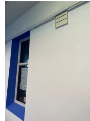
Flat 84 Foundling Court 1 additional grills
