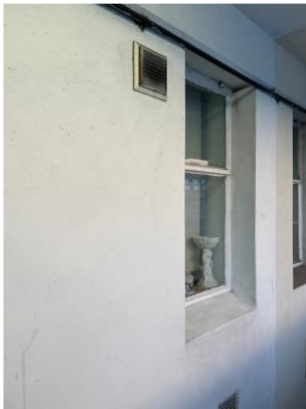
Flat 83 Foundling Court 1 additional grills
