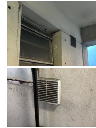
Flat 25 Foundling Court 2 additional grills
