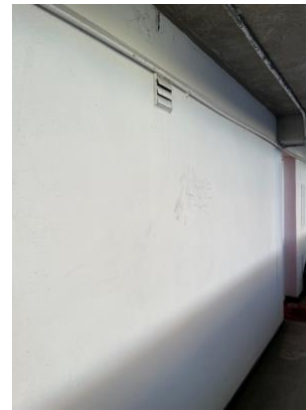
Flat 142 Foundling Court 1 additional grills
