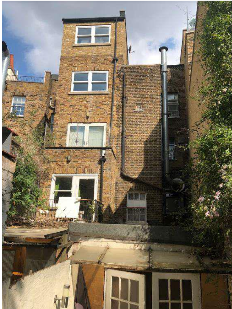
Figure 3: Rear elevation of application site. Existing extraction system visible on application site.
