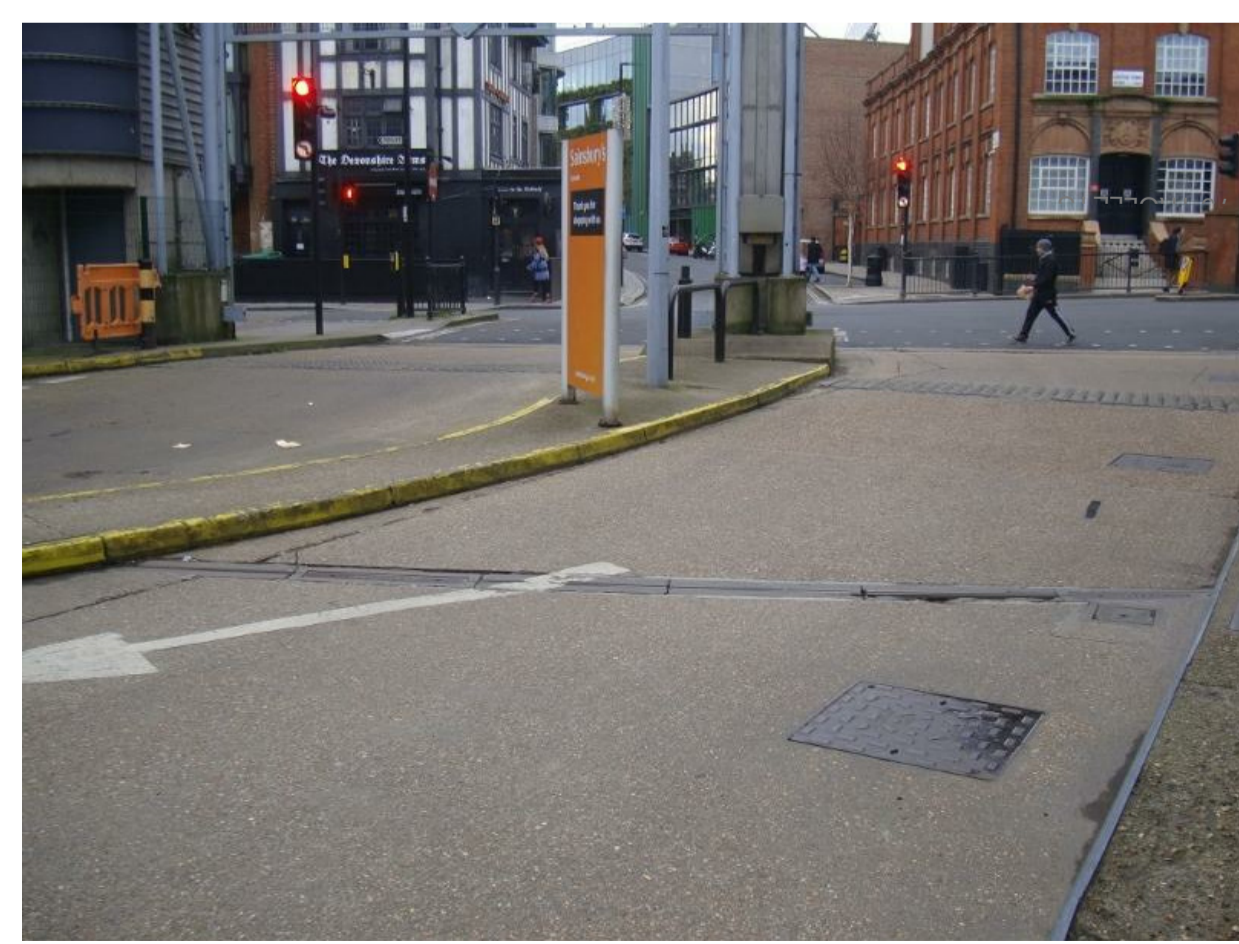
PHOTO 01 - SHOWING DAMAGE TO DRAINAGE (SCALE - NTS)
