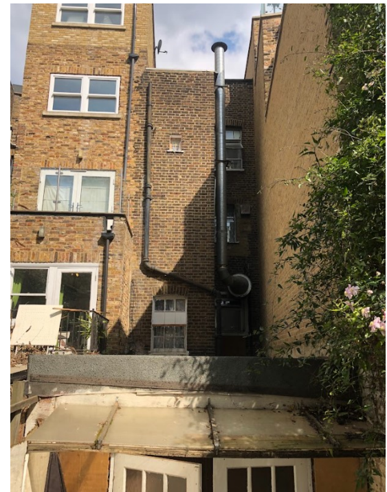
EXISTING EXTRACTION SYSTEM - EXTERNAL
