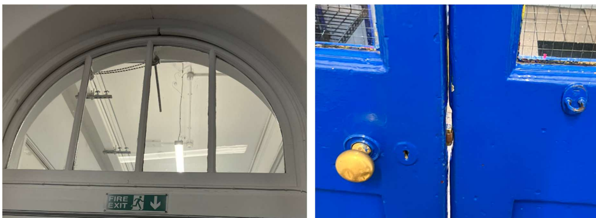
Figures 2 and 3: non fire rated glazing to be replaced & Damage to door leaf allowing passage of flames/smoke
