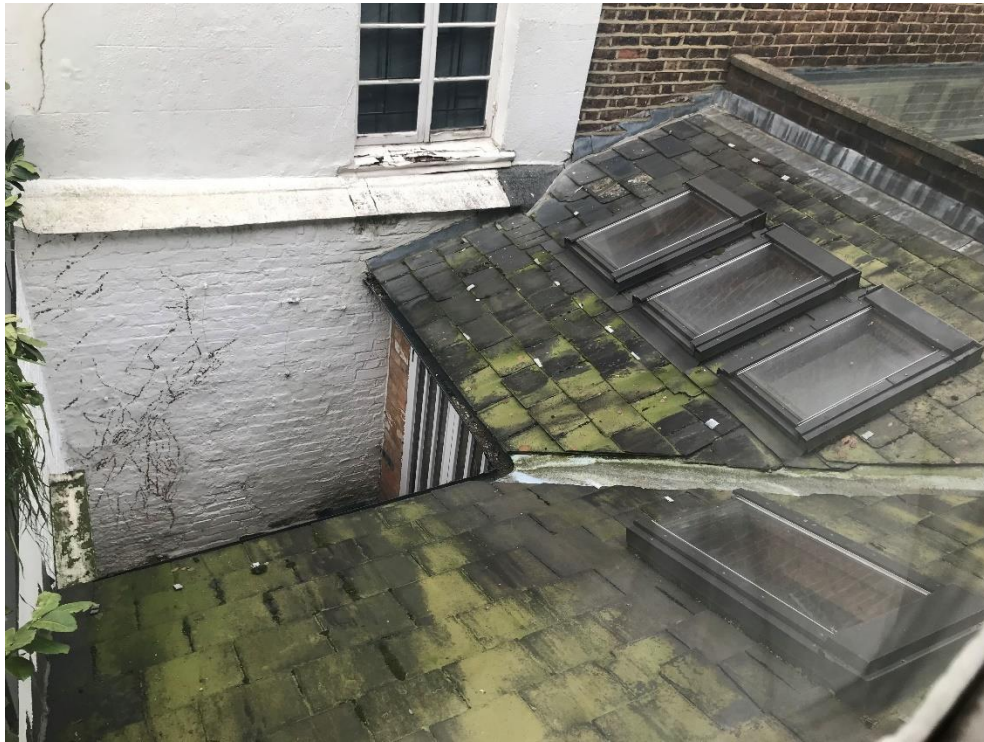
Figure 29: View of existing rear extension as built in 1987, seen from the staircase window.
