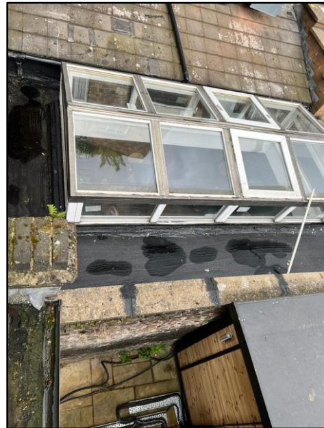
Figure 4 – Roof of conservatory to abutting property (photo taken from outbuilding in question).
