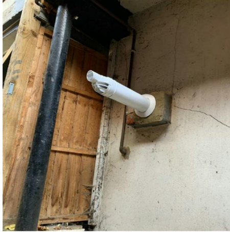
Lower ground falt - cracking above door at rear junction
