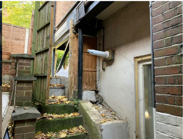
Supporting column to original projection and diagonal crack on lower ground flat wall
