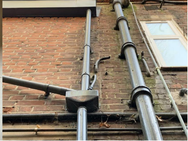
Cracking at junction on left flank wall
