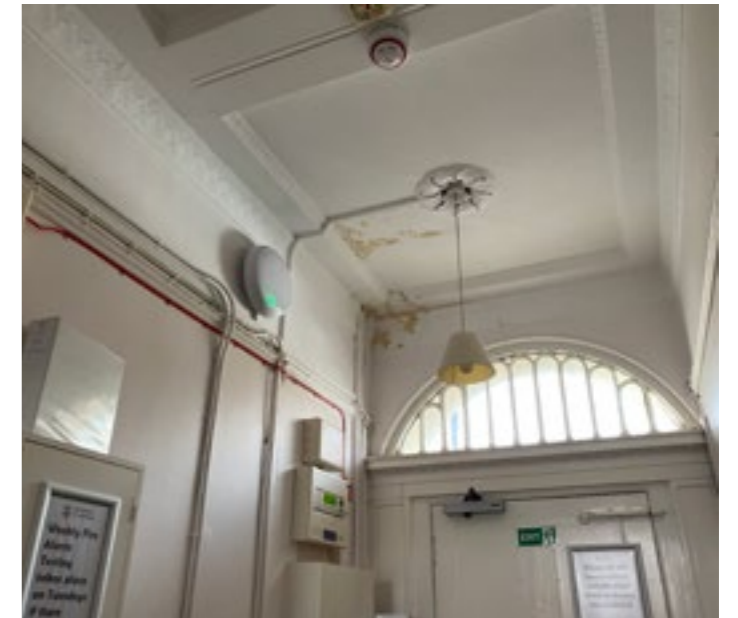
Figure 5.6 Main Entrance services
