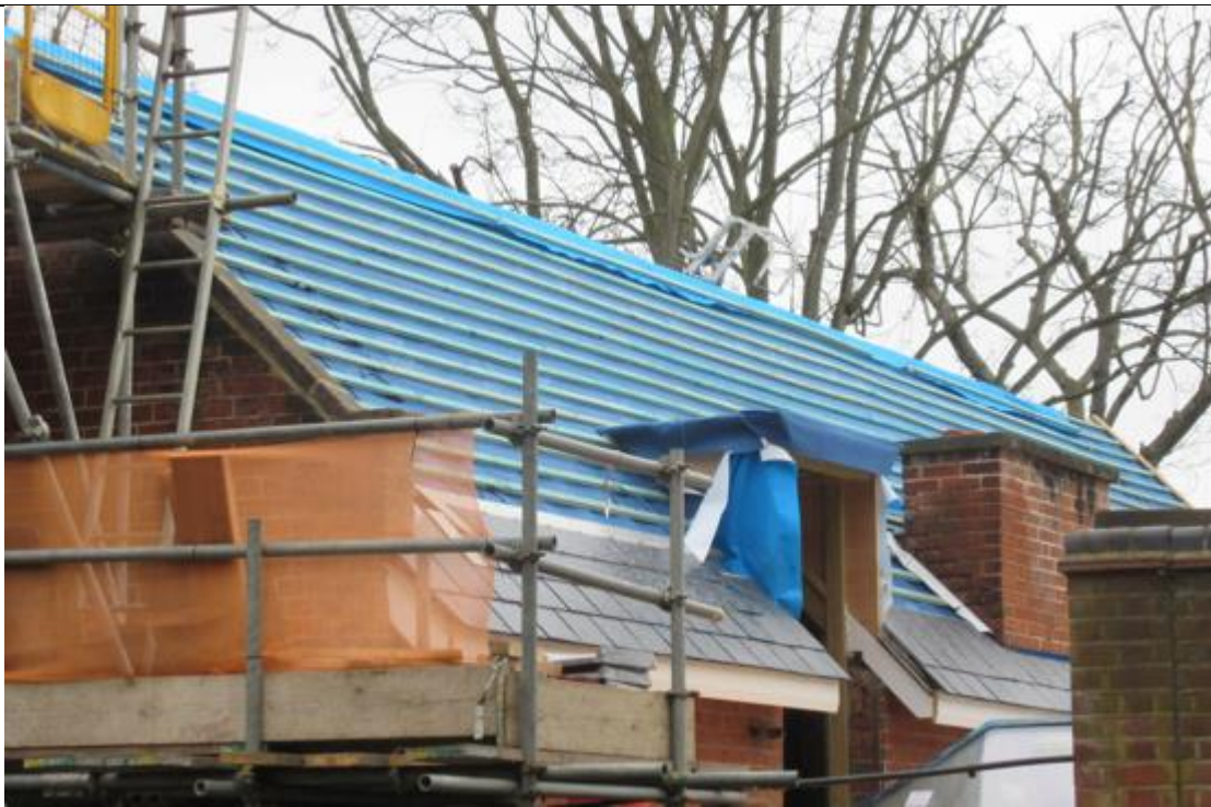
Figure 3: Photo from site visit showing the solar and unoriginal grey slates being fixed to the roof
