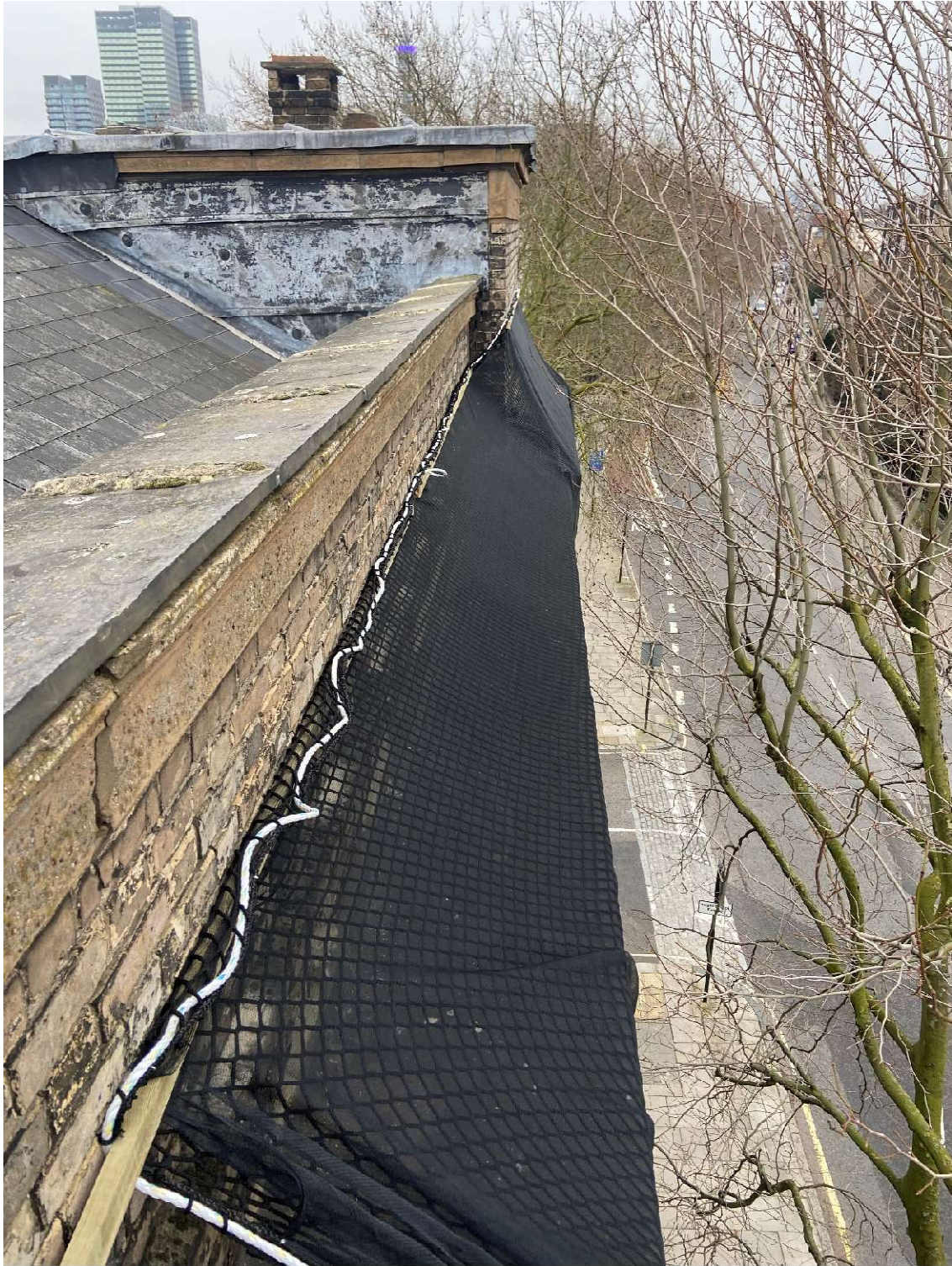
Img. 2; Close-up view of black netting installed to sky-facing edge of cornice
