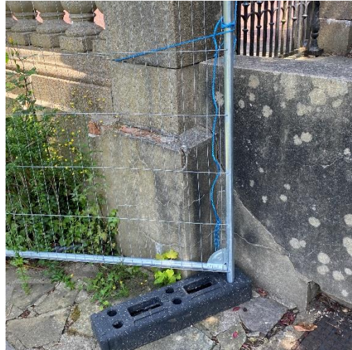
Figure 10 Cracking at wall low level
