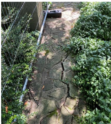
Figure 13 Stress fractures through paved pathway from tree roots
