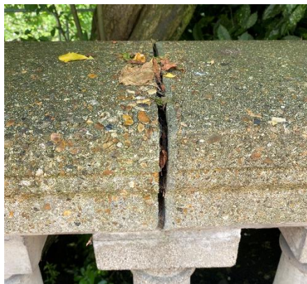
Figure 7 Open joints between coping stones
