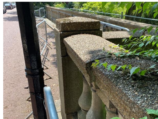
Figure 8 Dislocation of coping stones -able to be moved by hand
