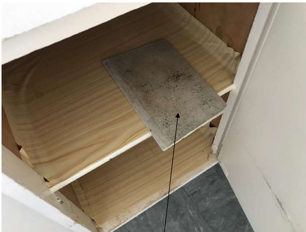
Loose Panel on Shelf
