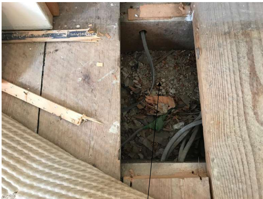
Debris Under Floor
