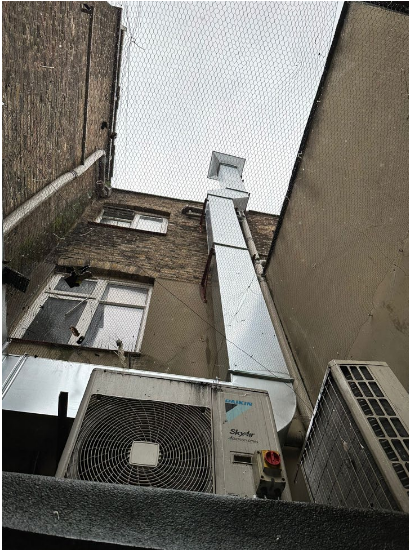
Photo 1 View of exhaust ductwork from yard
