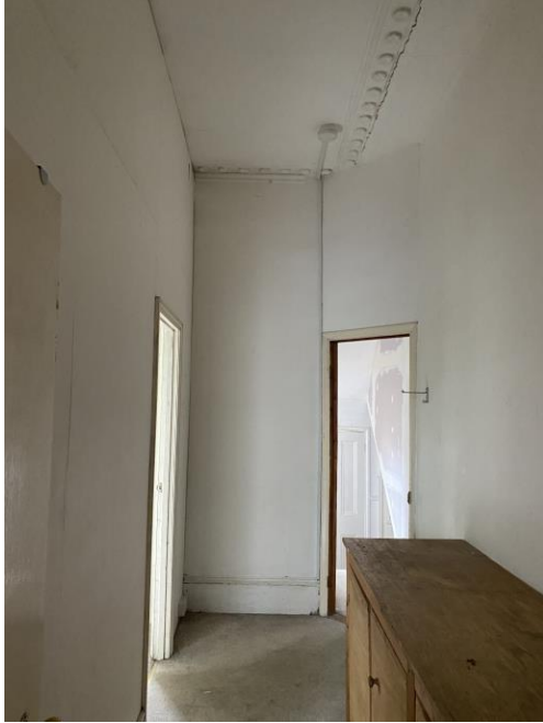
Figure 28: Corridor created out of rear room with original cornice evident on right hand side.
