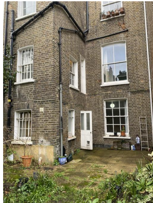
Figure 27: Rear elevation with windows and doors to outrigger. This shows the redundant doorway that disrupts the composition of the rear elevation.
