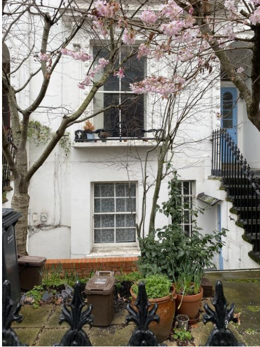
Figure 29: Front elevation with poor retaining wall treatment.
