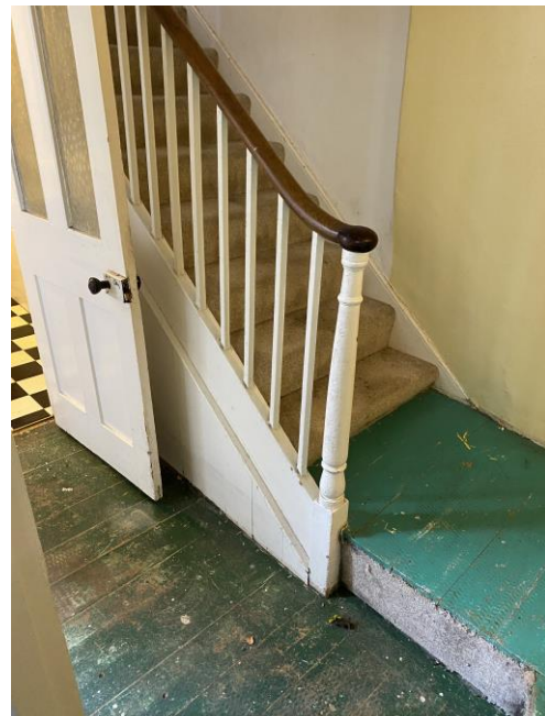
Figure 17: Original stair with bottom step altered from LGF.
