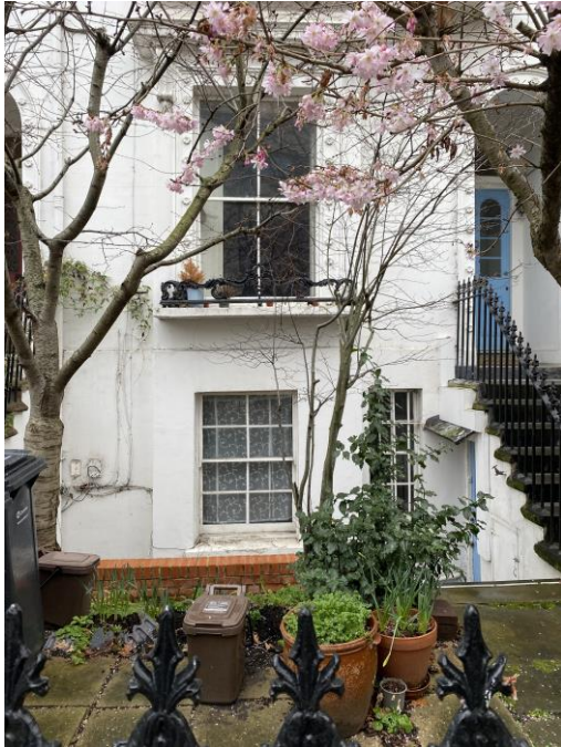
Figure 29: Front elevation with poor retaining wall treatment.
