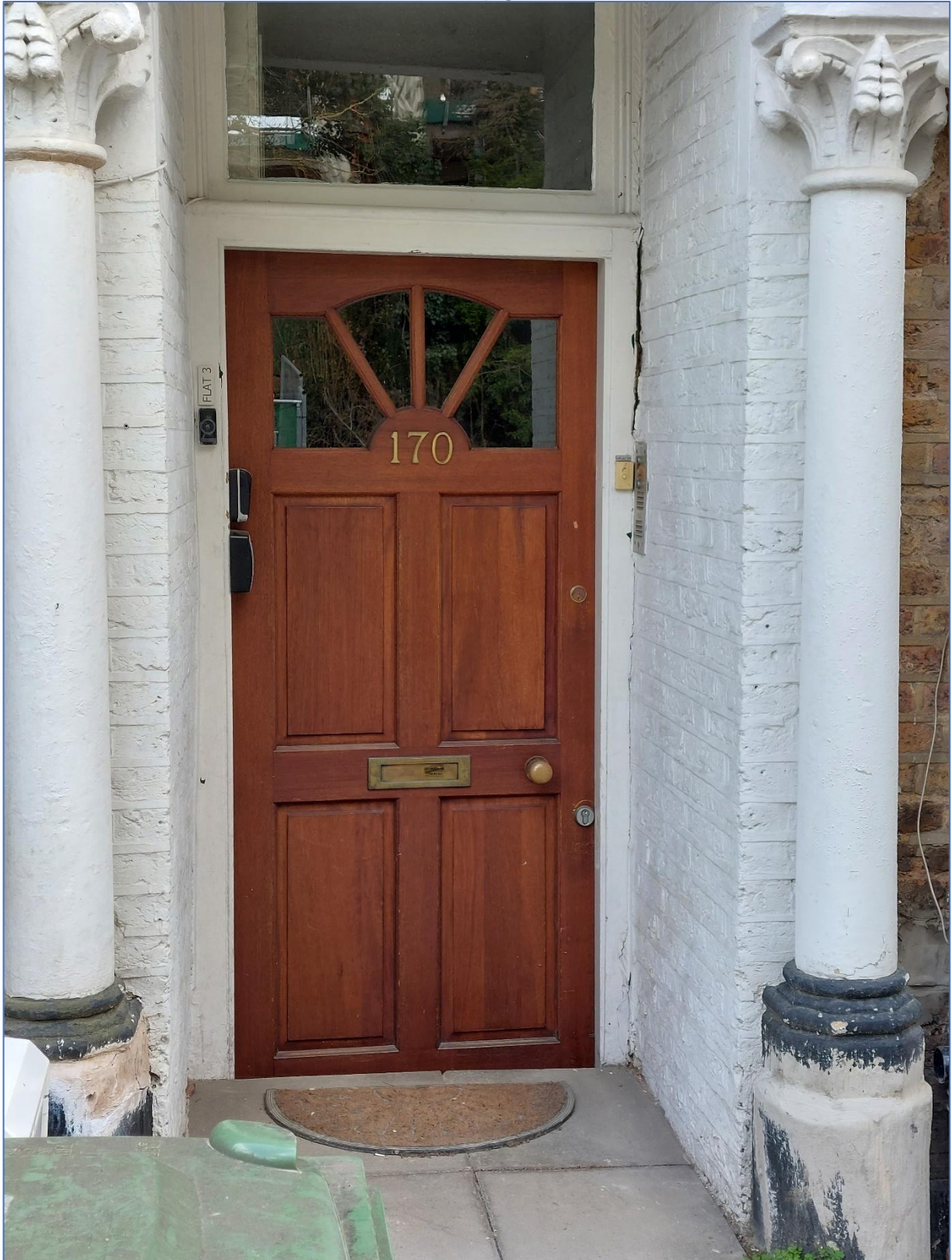
Photo 6: Front door with distortion and cracks around frame, claim address
