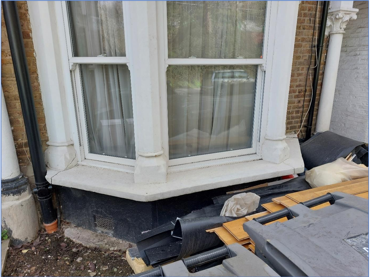
Photo 4: Cracks in bay window structure, claim address
