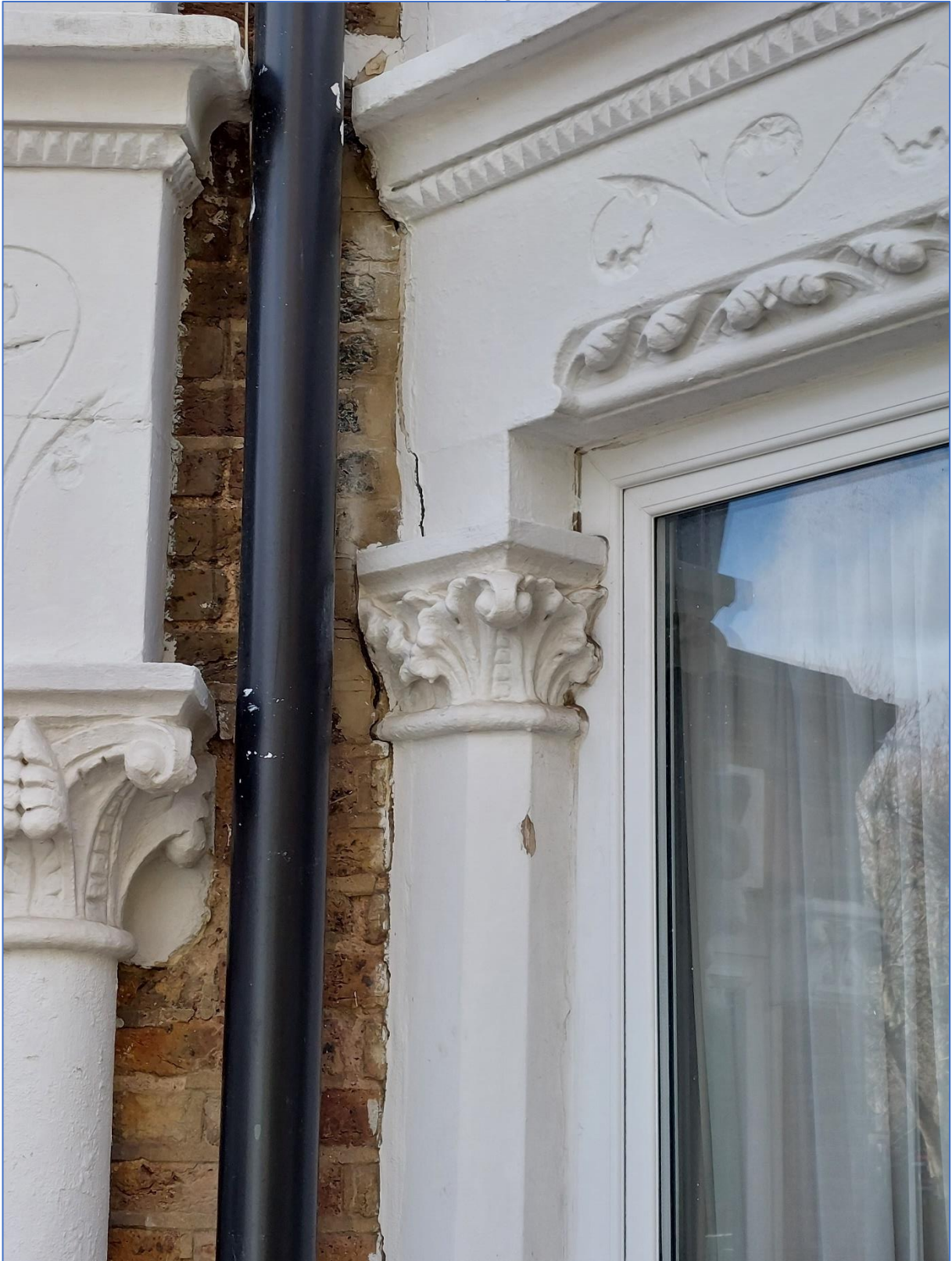
Photo 5: Cracks in window surround, claim address
