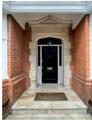
Existing Main Entrance to the House with hidden away limestone doorway surround
