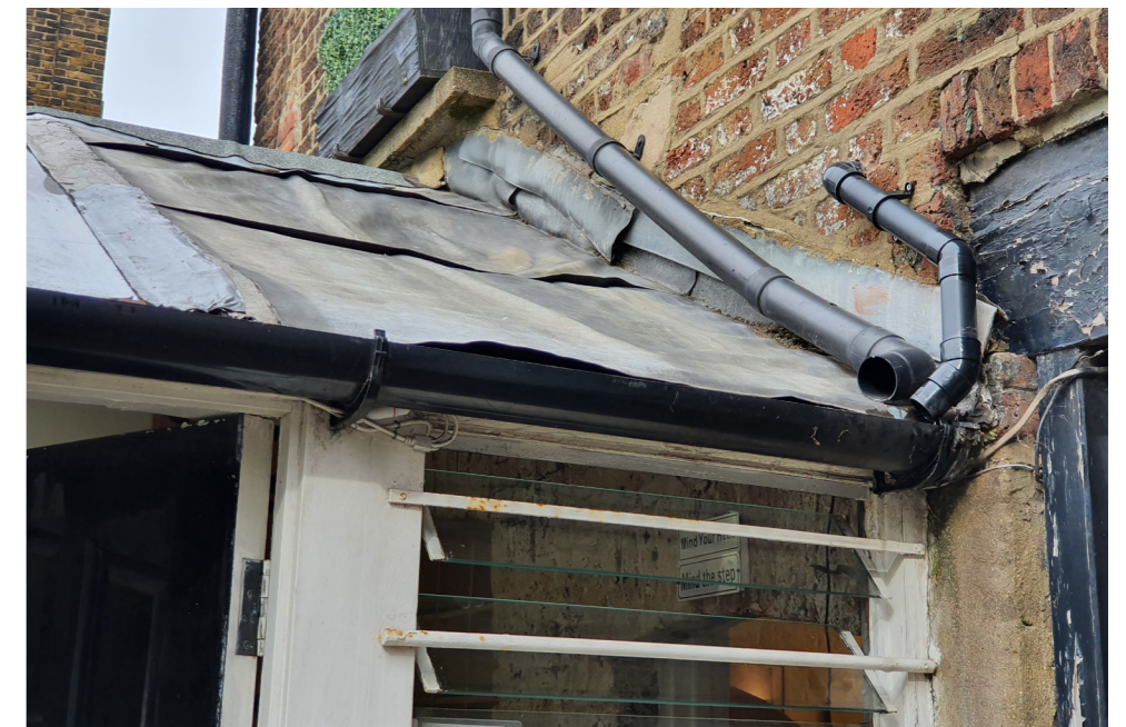
Ad-hoc nature of existing roof to annexe
