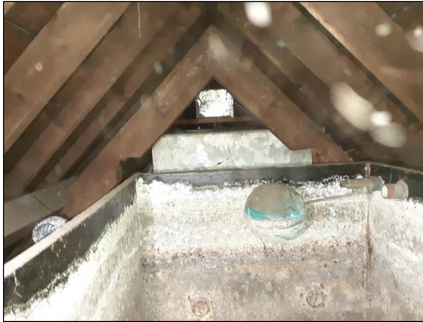
Fig 3 View of roof void within northern part of Building A (looking west from the eastern gable). The water tank in the foreground is empty and showed no evidence of bats
