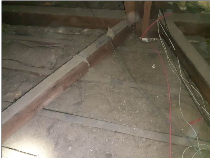
Fig 4 Floor of roof void within Building A. As with all the roof voids, characterised by a significant layer of detritus.
