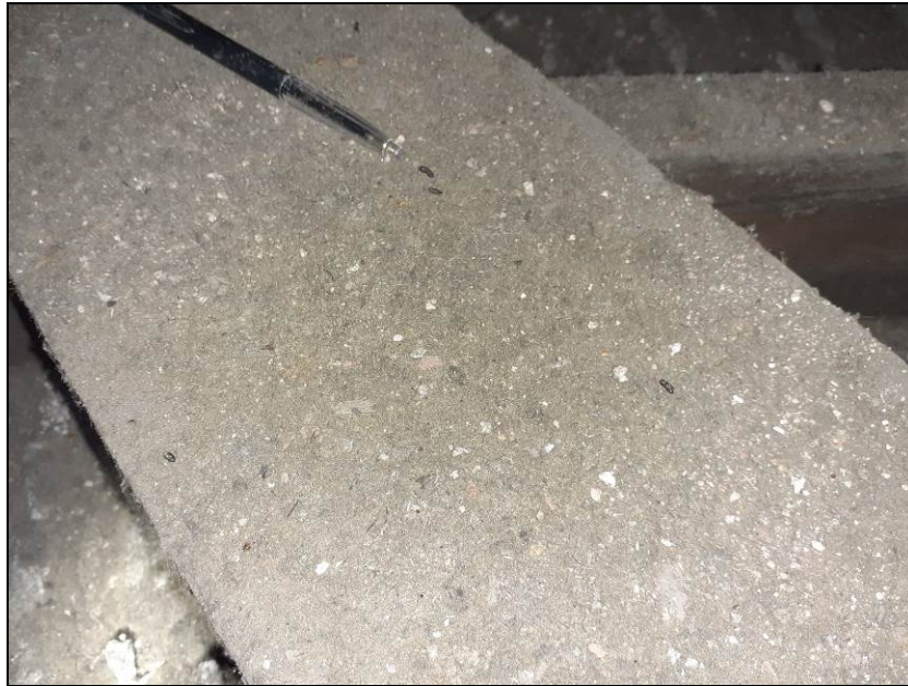
Fig 8 Bat droppings on a loose plank in the roof void of the dormer on the east elevation of Building B
