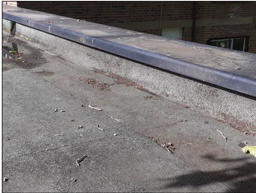
Fig 13 Roof of Wathan Hall. Felt in sound condition with no gaps. Coping to parapets has a gap along the length under the return, on both sides of the wall.
