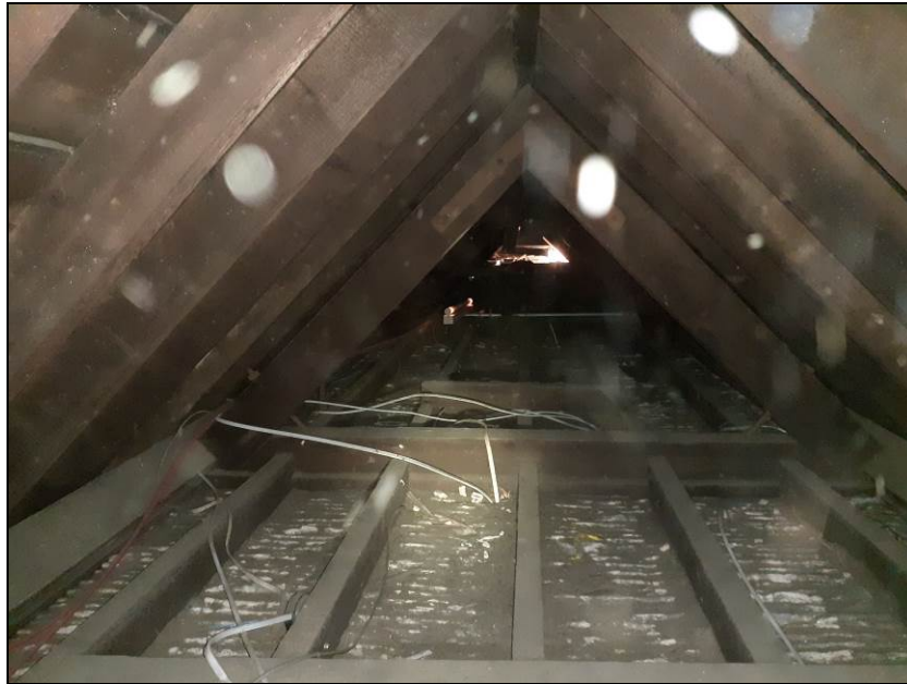
Fig 5 Roof void within Building B (looking north from the southern gable). The lath & plaster ceiling and timberwork are covered in detritus.
