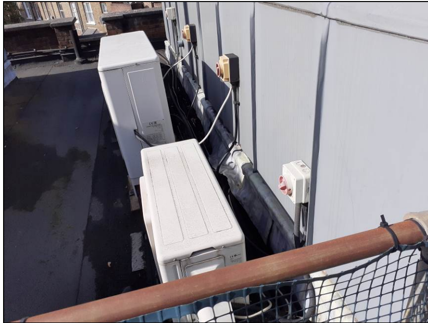
Fig 11 Lifting lead flashing (centre of photograph) to the base of the 'pods' on the flat roof of Building C.
