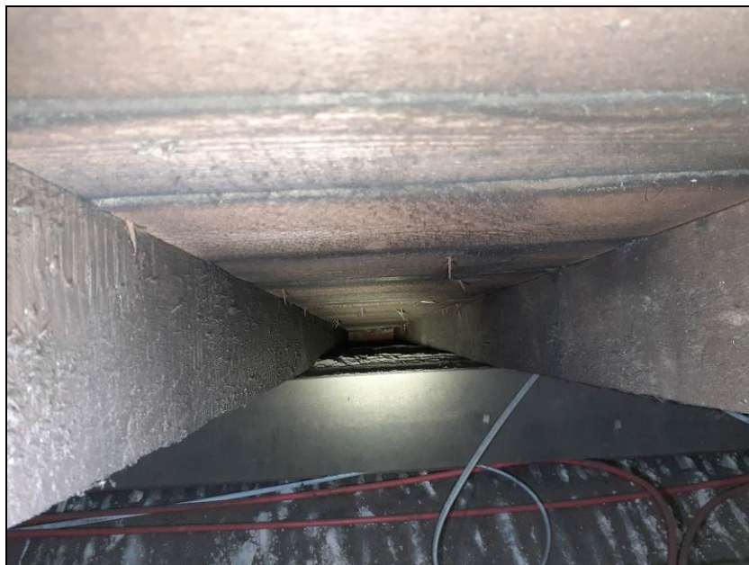
Fig 6 Gap between the sarking-clad pitch and the hip of the roof extending down to the eaves
