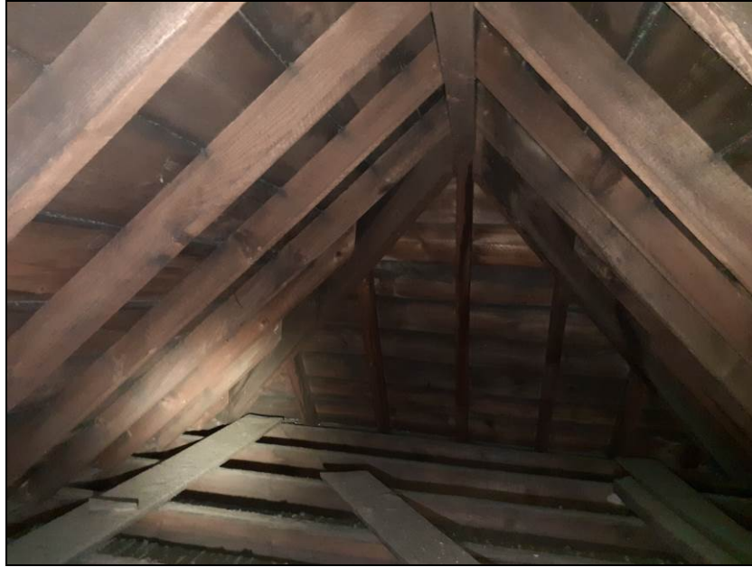
Fig 10 Loose plank of timber within the eastern dormer of Building B. No staining or evidence of roosting was noted associated with the timbers above.
