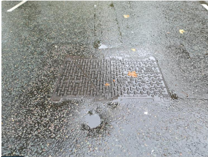
2 G.Network Chamber, close up view
