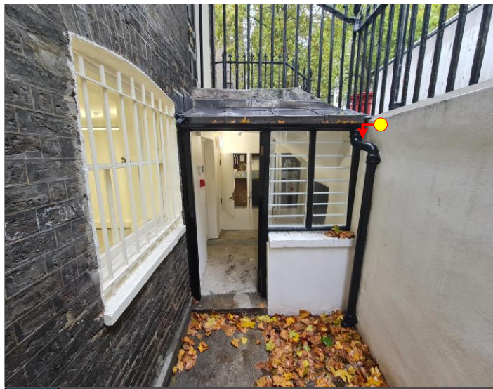
9 Multicore cable route, to existing FSB
