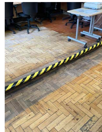
flooring needs repair
