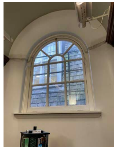
Existing windows in need of repair
