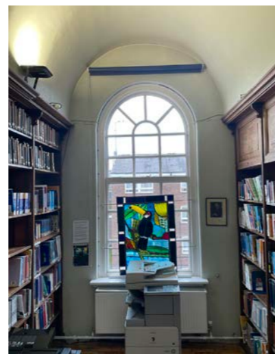
Existing windows let in noise and sunlight
