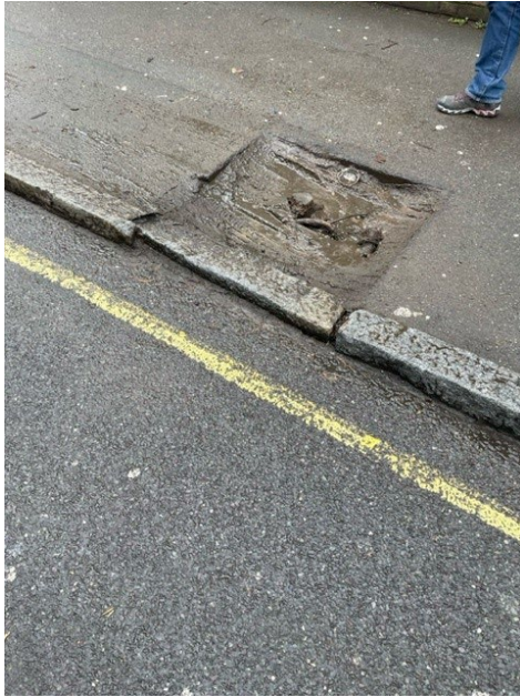
Existing damage caused by Mulalley opposite entrance
