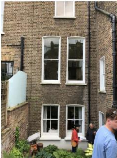
rear elevation showing existing large GF sash windows and smaller LGF sash windows
