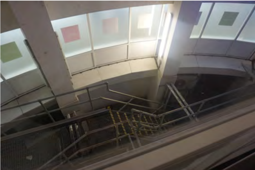
56A Tower block mixed mode ventilation duct with modern infill (Insall)
