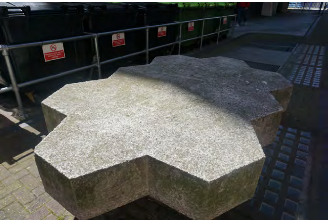
48B Original forecourt concrete extract cover (Insal)
